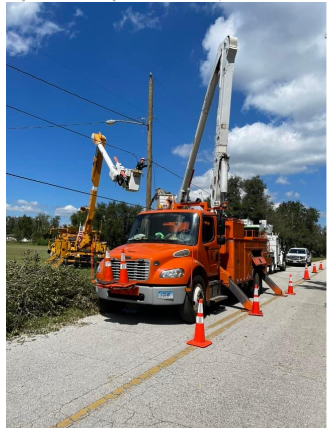
Wallingford Electric Division Crew Restoring Service in Bartow Electric service territory in Florida after Hurricane Ian
