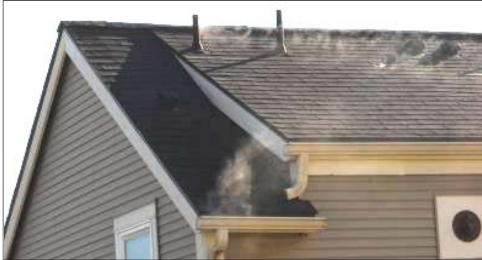
Smoke testing of the stormwater system in the New Holly development in Seattle identifies a home with an illicit connection.
